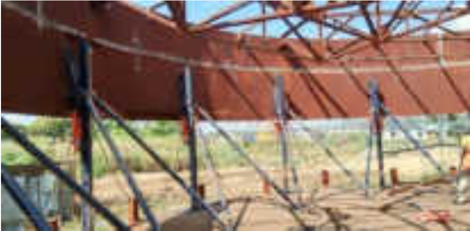
Storage Tank with Jack system
