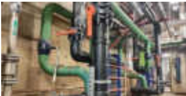
Water Piping systems
