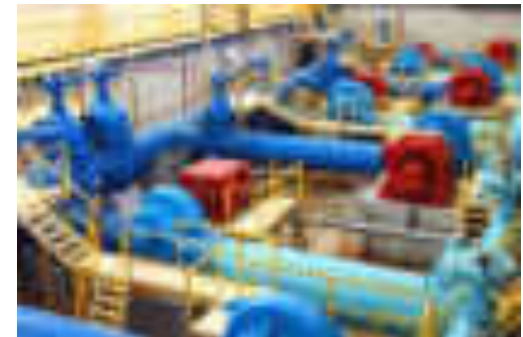
Sea water pumping house
