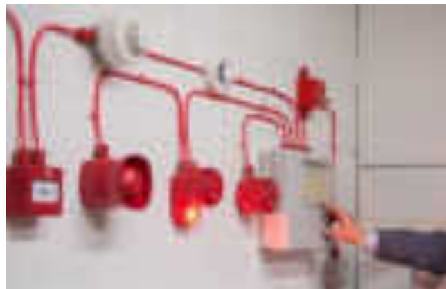
Fire detection and Alarm System
