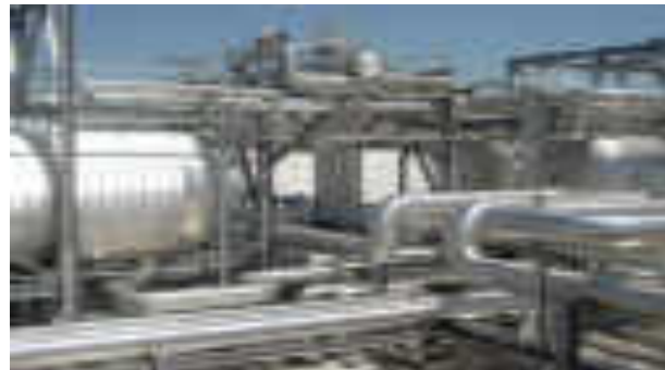
Steam Piping systems
