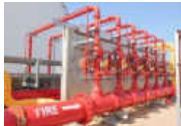
Fire Protection System
