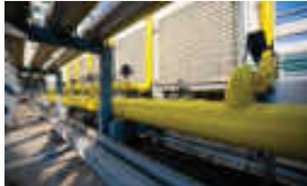
Chilled and cooling water piping system
