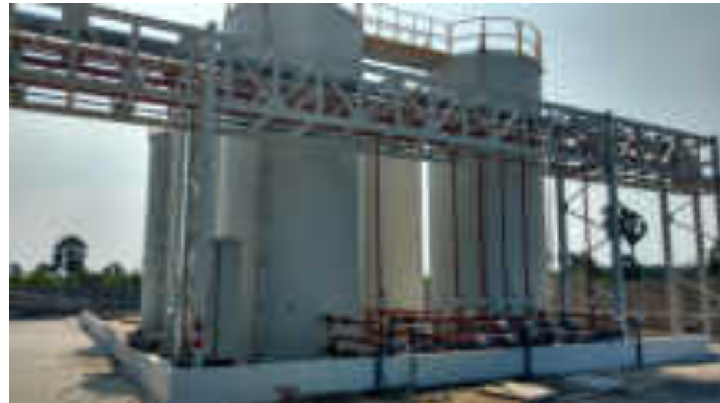
Tank Farm with Truck Loading Systems
