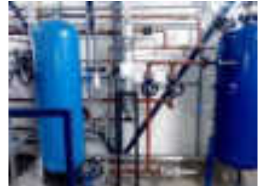
Gas piping system
