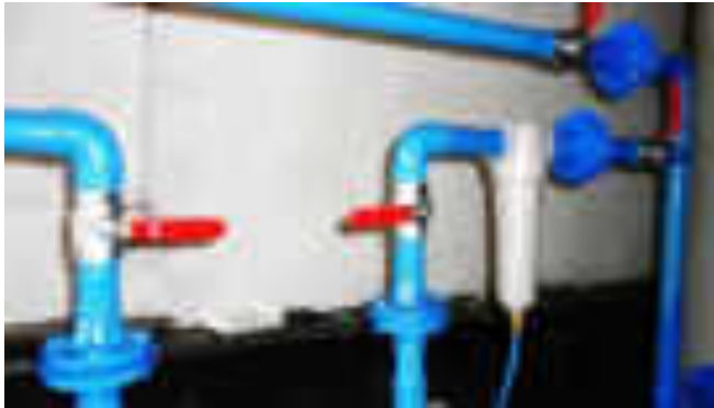
Compressed Air Piping
